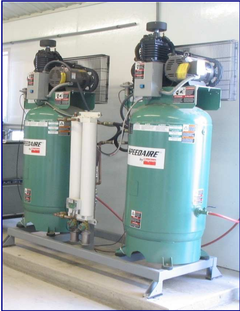
(2) 5 hp Speedair Compressors , modularized;
