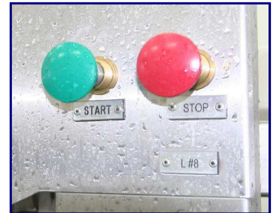
Left: Main Control station in back of parlor;
