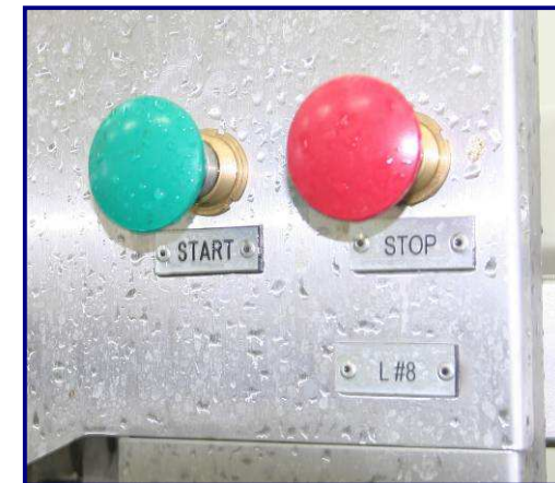
Left: Main Control station in back of parlor;
