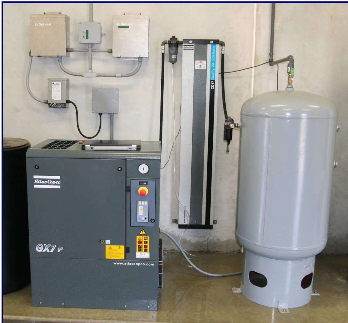
(10) hp Atlas-Copco Screw Compressors
