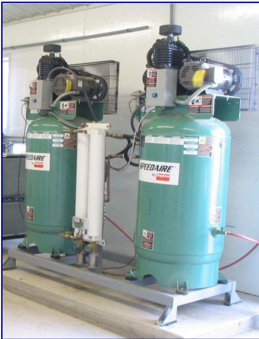
(2) 5 hp Speedair Compressors , modularized;
