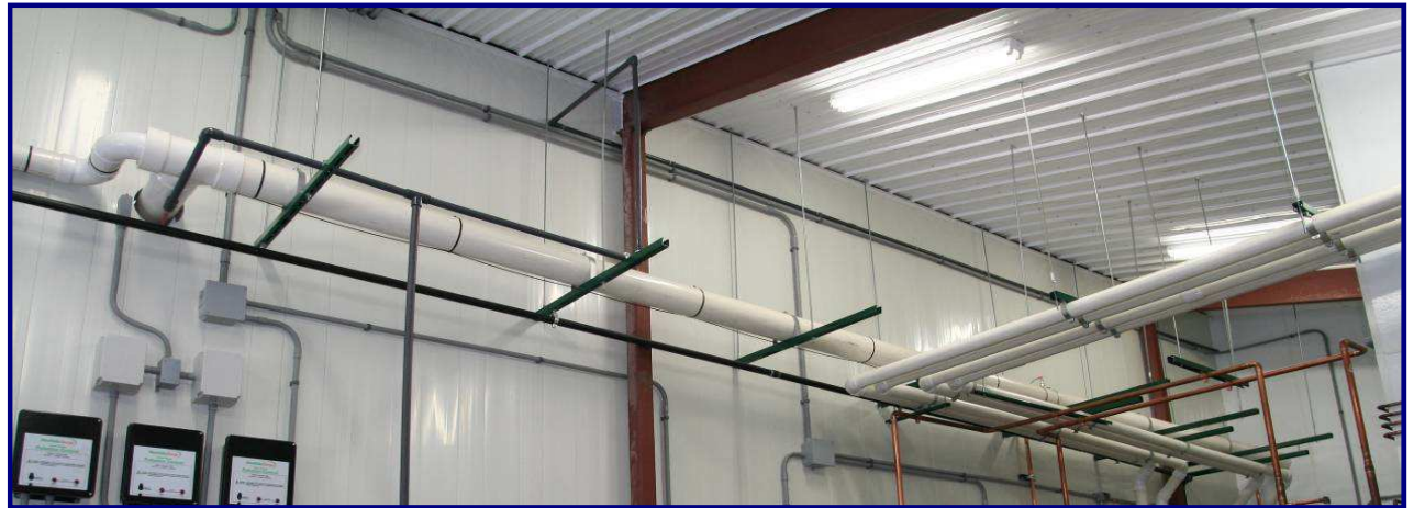
6" Header Line supplies CIP Receiver Group and Pulsation System
