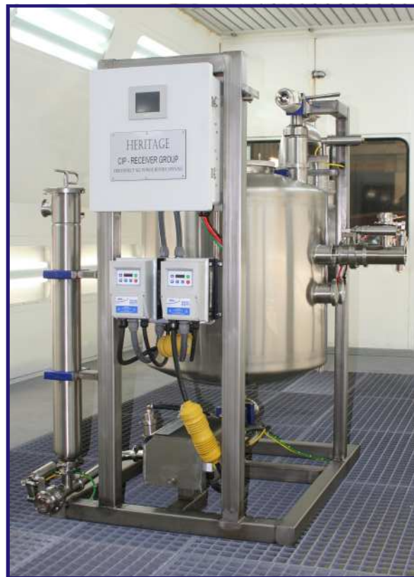
HERITAGE Model 1500 CIP Receiver Group installed at Steve Paul's new dairy, Whitewater, WI, where it supports an all-stainless dbl. 10 (expandable to dbl. 16) HERITAGE ProTime I HerringBone with Arm TakeOffs
