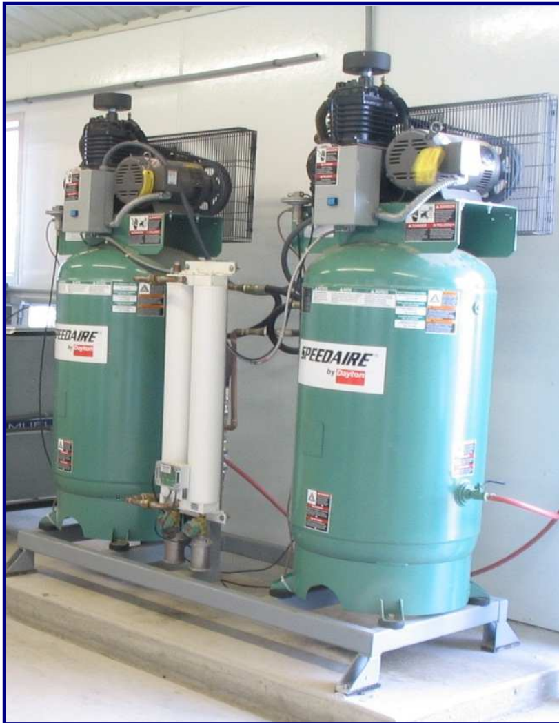
(2) 5 hp Speedair Compressors , mod# 44 of 33
