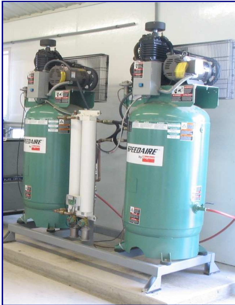
(2) 5 hp Speedair Compressors , modularized;
