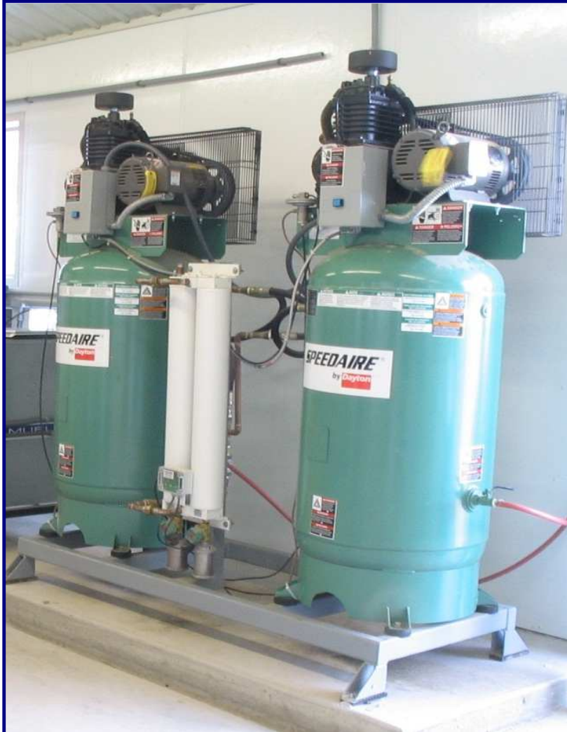
(2) 5 hp Speedair Compressors , modularized;
